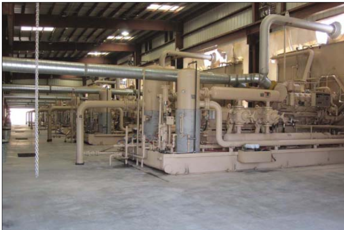
Two-stage reciprocating compressors increase the gas pressure to the gas plant inlet pressure of 800 psi from the 250 psi in the gathering line (Fig. 6). Photo by Guntis Moritis.
