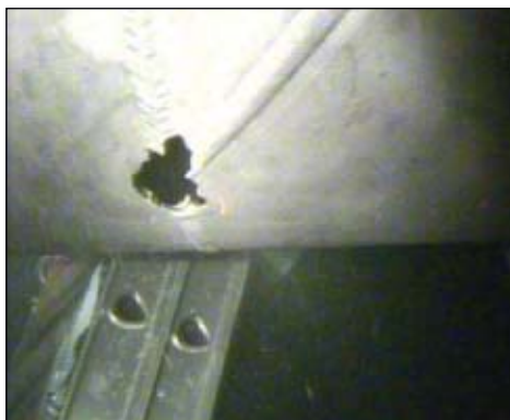
This leak hole lies at the weld junction of the Forties Bravo to Forties Charlie 20-in. OD pipeline (Fig. 1).
