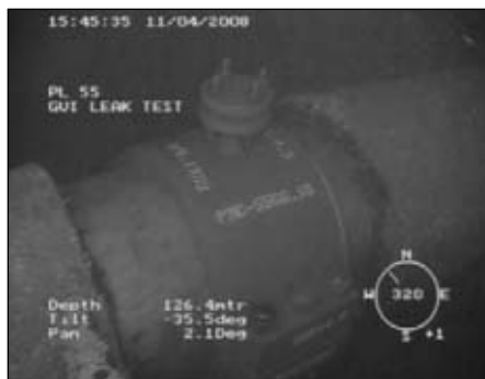
Installation of this clamp as repair to the weld junction of the Forties Bravo to Forties Charlie pipeline took a total of 6 days following detection of the leak (Fig. 2).
