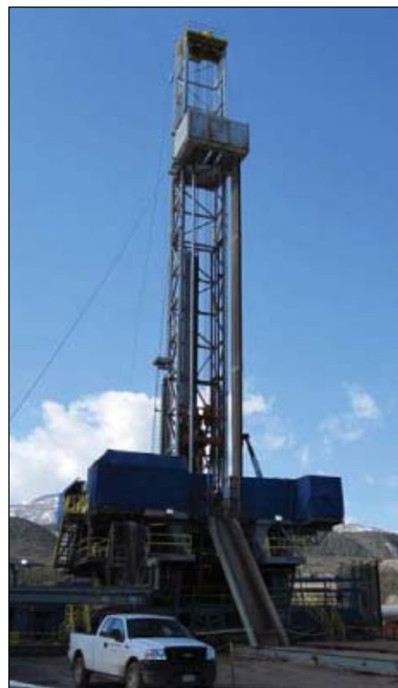
The H&P Flex Rig 278 on this well pad in South Rulison field will drill 22 wells (Fig. 1). Photo by Guntis Moritis.
